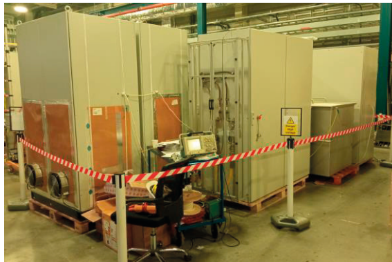
Figure 9.3: Overview of prototype converter chain including high-voltage oil tank assembly and load cabinets. Three resistive load cabinets are obscured by the low-voltage cabinet.
