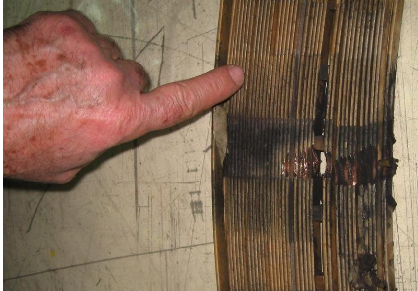
Figure 105: Exact location of the internal turn-to-turn fault in phase L2.
