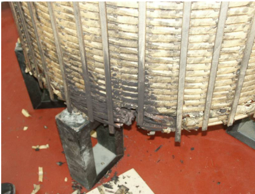
Figure 101: Common auto-transformer winding internal fault in phase L3 at the winding neutral point.
