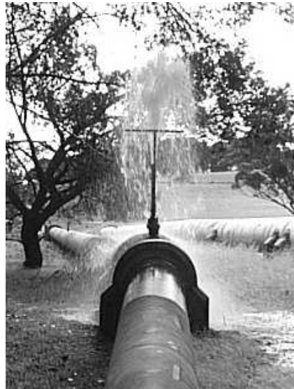
Figure A.13: Artificially generated leak
