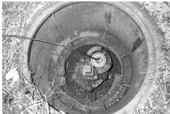
Figure A.9: The connected fire hydrant cap with incorporated transducer.
