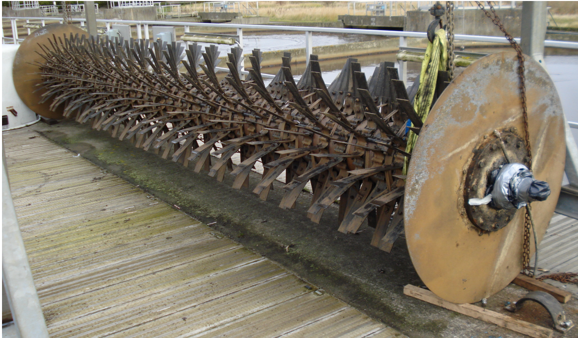
Figure 6: Surface aerator used at Avedøre WWTP
