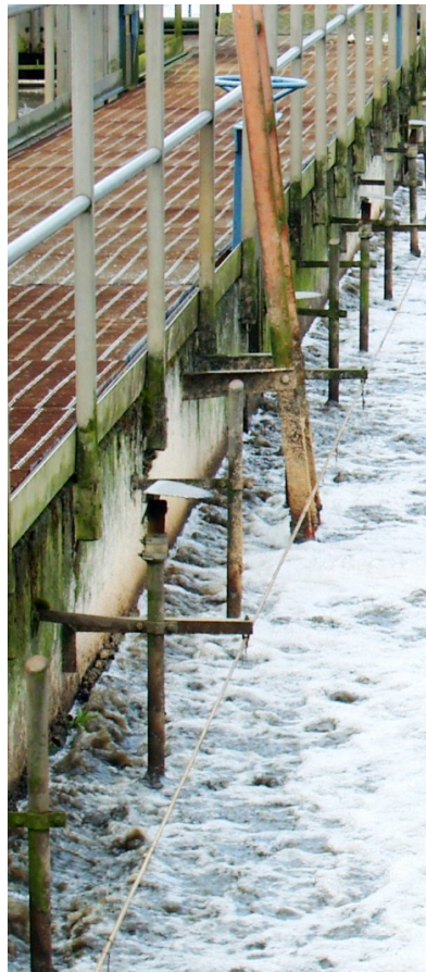
Activated sludge process at Sjölanda.
