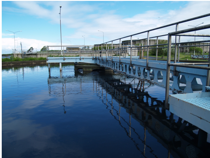
Figure 3.1 Primary sedimentation basin
