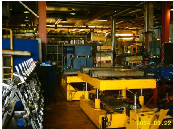
Figure 16: Carriage for loading press tools.
